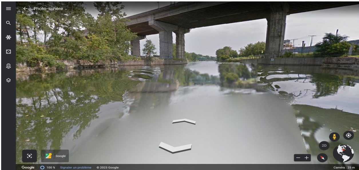
Picture 6c - Obstacle (O2) of the Route 138 overpass - View from the water - Direction Start
